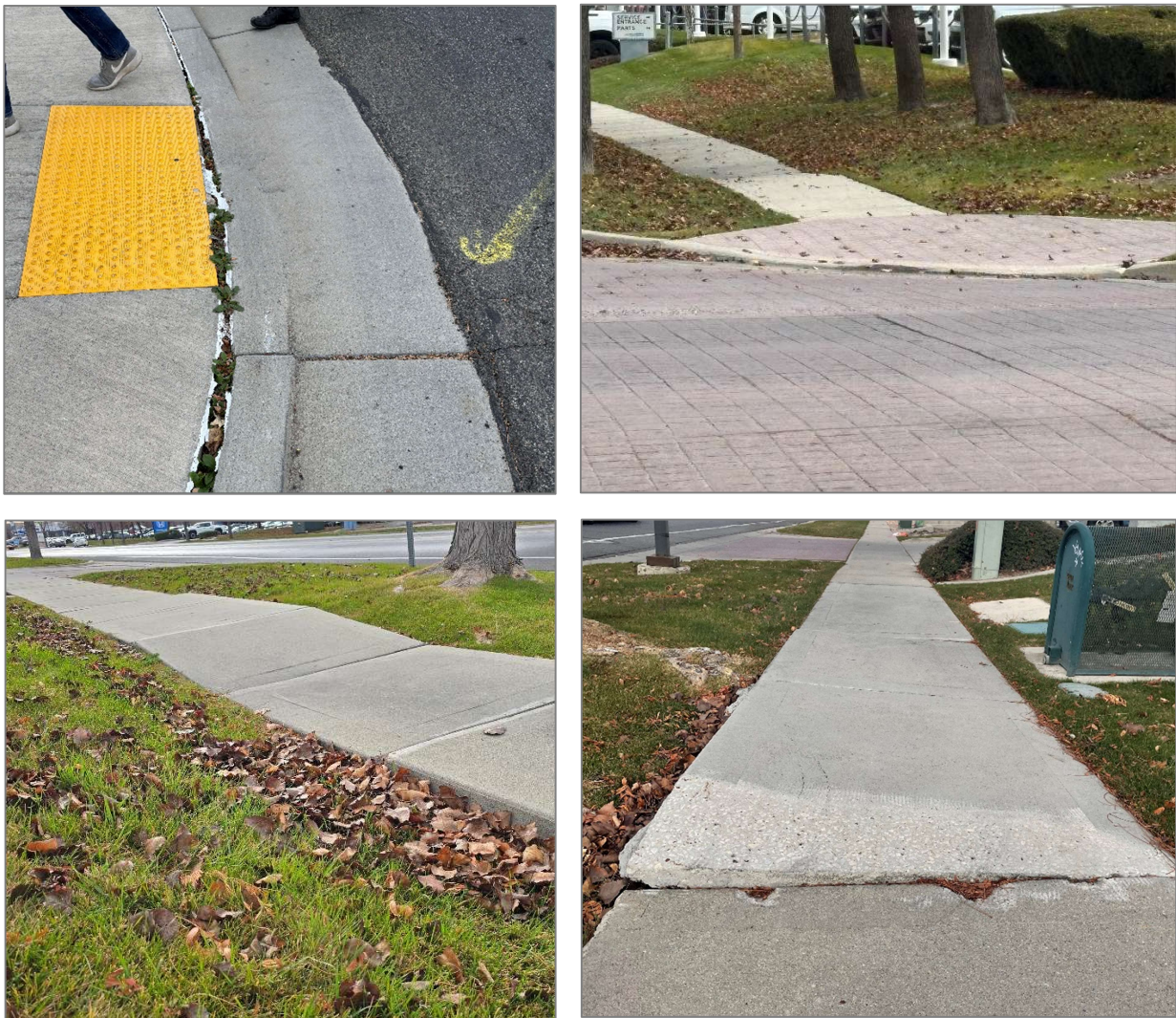
Figure 10: Sidewalks are uneven in places and ramps are not all ADA-compliant
